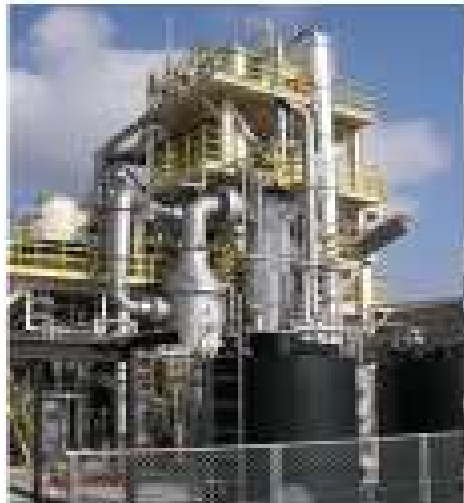
HyPR-MEET demonstration plant
