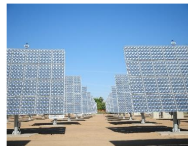
Courtesy: CPV Installation at Nichols Farm
